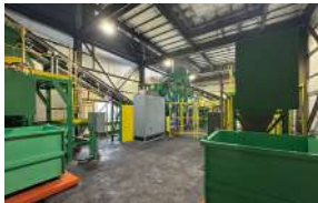
Tire shredder (Miyazaki Factory)
