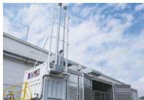
Hydrogen production unit (Shirakawa Factory)
