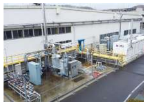
Hydrogen production unit and hydrogen boiler system (Shirakawa Factory)
