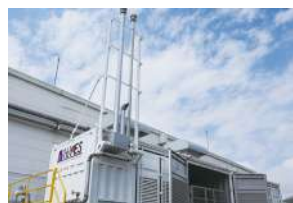
Hydrogen production unit (Shirakawa Factory)
