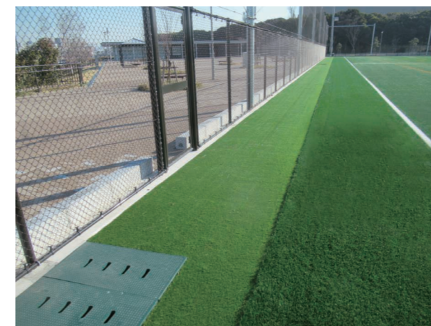
Water-permeable artificial turf is installed on the rainwater ditch to filter microplastics, and blocks are installed around the field to prevent microplastics from scattering by wind.
