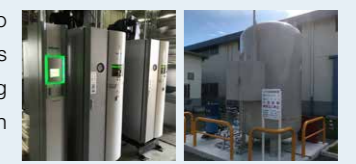
Ono Factory boiler and LPG tank
