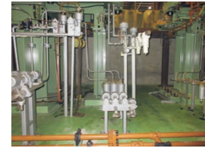
Steampipe drain pocket installed at Hunan Factory (China).
