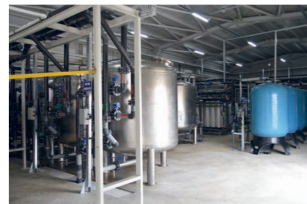
Wastewater recycling facilities (Turkey Factory)
