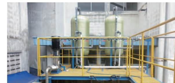
Rainwater utilization system (Indonesia Factory)
