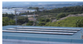
Solar panels installed in the Ono Factory of Dunlop Retread Service Co., Ltd.
