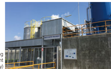
Wastewater recycling equipment (Thailand Factory)
