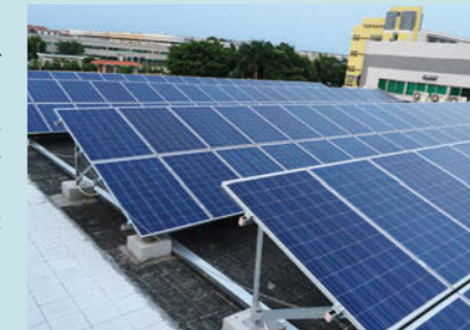
Installed solar power generation system
