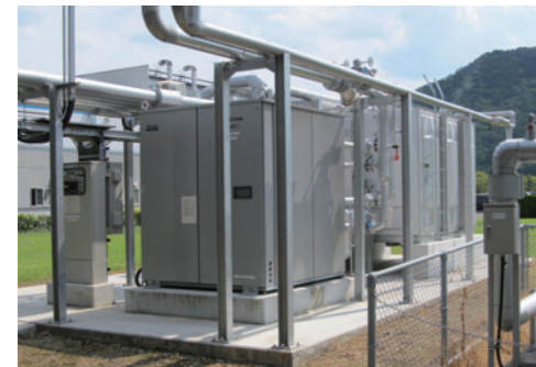
Waste-heat recovery equipment at the Ichijima Factory
