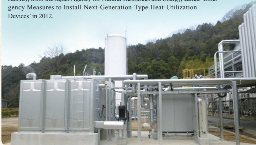
Hot water absorption chiller and hot water storage tank
