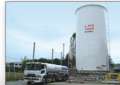
Just completed, this is one of the largest LNG satellites in Japan
