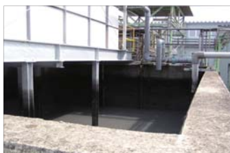
Wastewater treatment facilities
