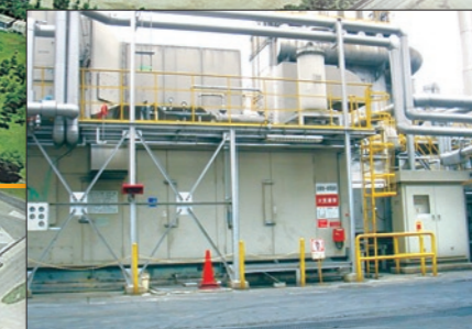
Shirakawa Factory cogeneration system
