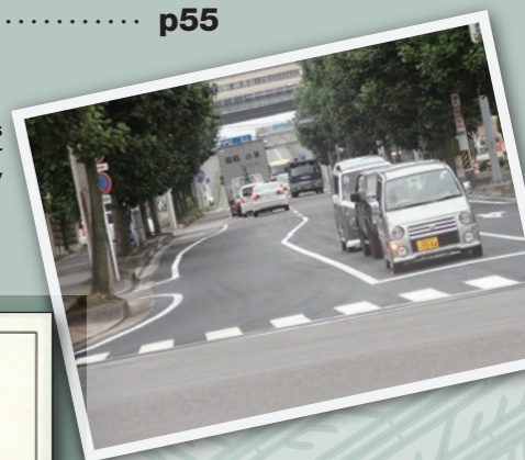
Making effective use of old tires by using them to make asphalt-rubber for a road in Shirakawa City
